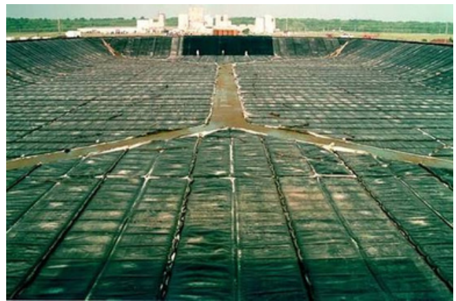
The LemTec gas collection system was specifically designed to work with wastewater treatment ponds, enabling biogas collection and fuel use in multiple countries.
